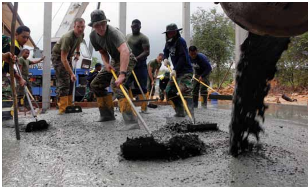
Marines and sailors with the Royal Thai Navy and Indonesian service members spread concrete over a foundation at the Ban Khlong Bangbor school in Rayong, Thailand, Jan. 20 as part of humanitarian and civic assistance projects that precede the official kickoff of Cobra Gold 2012. "Through humanitarian and civic assistance programs, we have an opportunity to support the needs of our friends and regional partners," said Lt. Gen. Kenneth J. Glueck Jr., deputy commander of CG 12 and commanding general of III Marine Expeditionary Force. The Marines are part of Marine Wing Support Squadron 172, Marine Wing Support Group 17, 1st Marine Aircraft Wing, III MEF. Photo by Cpl. Jessica Olivas
