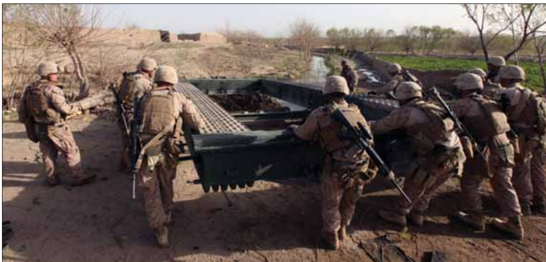
Marines slide a four-bay medium girder bridge across a canal in Mirmandab, Afghanistan, March 23. The Marines are with Company A, 9th Engineer Support Battalion, 1st Marine Logistics Group (Forward), and conducted an 11-day operation that called for bridges to be built and patrol bases to be established.
