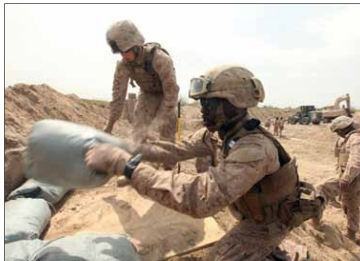
Lance Cpl. Corey J. Washington places sandbags in position on a newly established patrol base in Mirmandab, Afghanistan, March 29. Washington is a combat engineer with Company A, 9th Engineer Support Battalion, 1st Marine Logistics Group (Forward).
